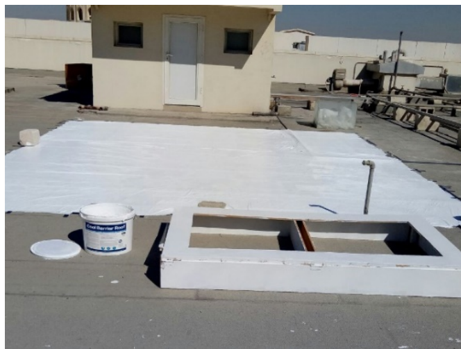
Figure 2: The cool carpet and rack #1 painted with the cool coating
